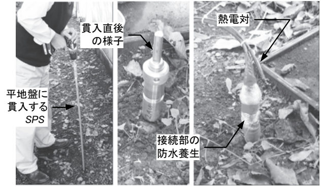
Photo 13 Installation of SPS for long term measurement.
