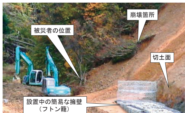
Fig. 1 Labor accident by slope failure in construction site. 斜面崩壊による労働災害の事例
