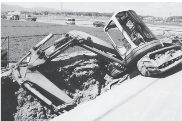
Photo 1 Ground collapse during trench excavation. 掘削中の建設機械の転倒事故の例
