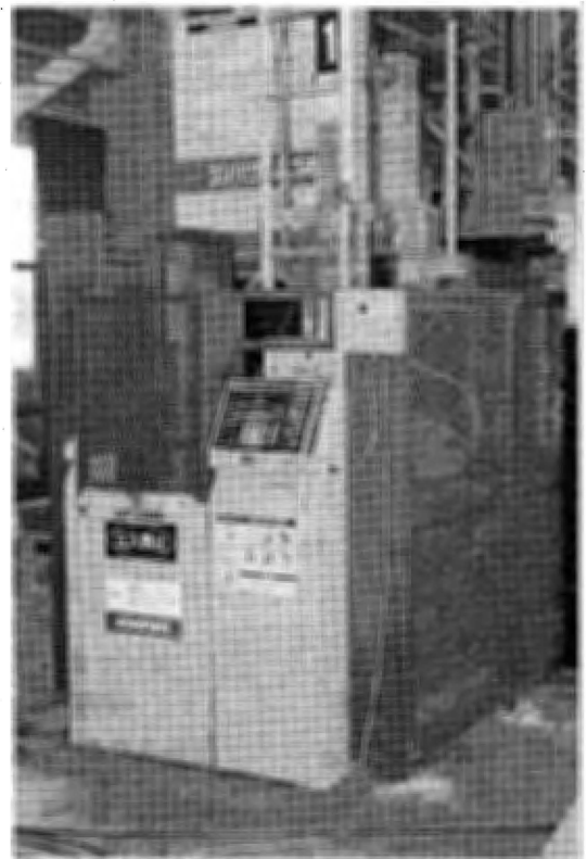
Photo 1 Guard for entrance to a danger zone. 危険領域の入口の防護
