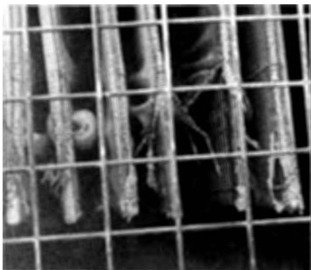
Photo 6-2 Damage of the filter cloths from an explosion.
