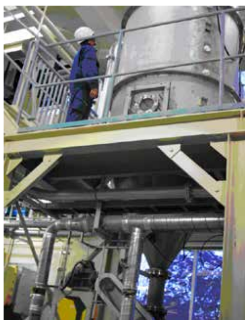
空気輸送粉体の静電気帯電・放電の調査 Pneumatic powder transport facility for investigating electrostatic charges and discharges.
